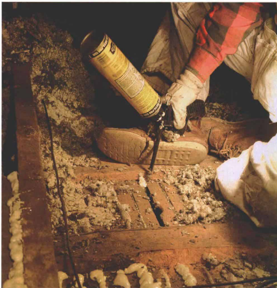
Smaller holes and cracks can be filled with caulk or foam. After attic insulation is pulled away, holes can be found and filled. Here the author fills cracks in a plaster-and-lath ceiling.
