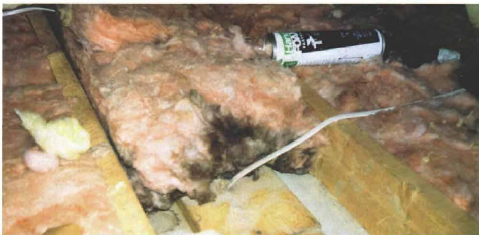
Dirty fiberglass signals an air leak. As warm air pours through penetrations in the ceiling, dirt is filtered out by fiberglass batts, but the heated air goes into the attic. Holes for wiring should be filled with expanding-polyurethane foam to stop the loss of this air.
